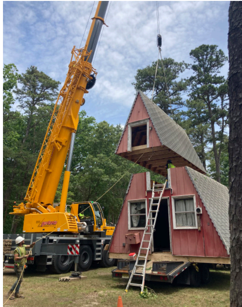
SJ Hauck Construction hoists the Triangle House into its new site. Photo courtesy Taylor Henry.
